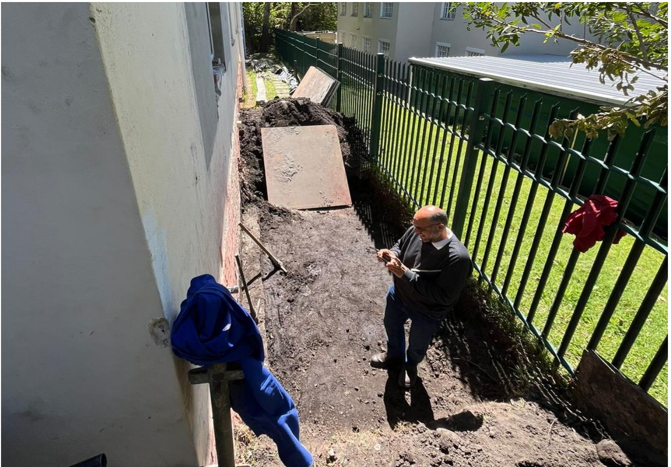
At the East side of the campus, prepping for the new sewer lines below the Old Hall
