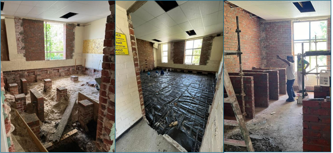
At the South entrance end of the Old Hall, 3 pictures taken a few days apart of the new bathroom floor and then the cubicles emerging
