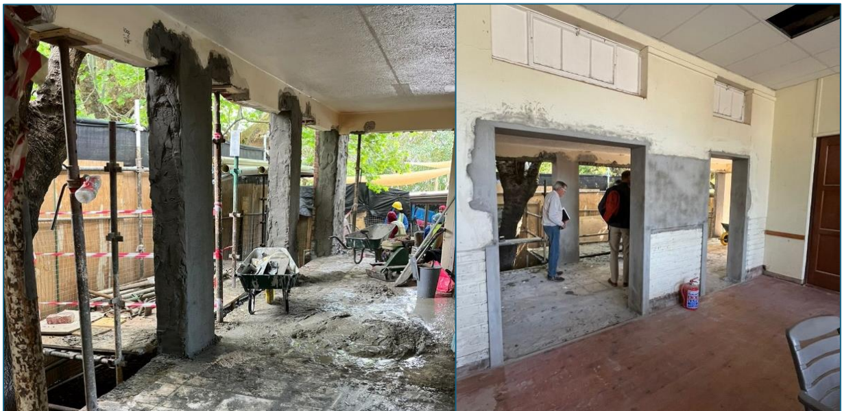
The old kitchen, now a covered walkway to access the garden and two new classrooms, from different angles
